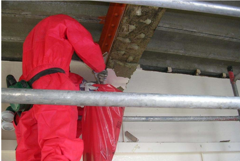
Figure 12.11 Bagging waste close to the point of removal to prevent spread and minimise exposure.
