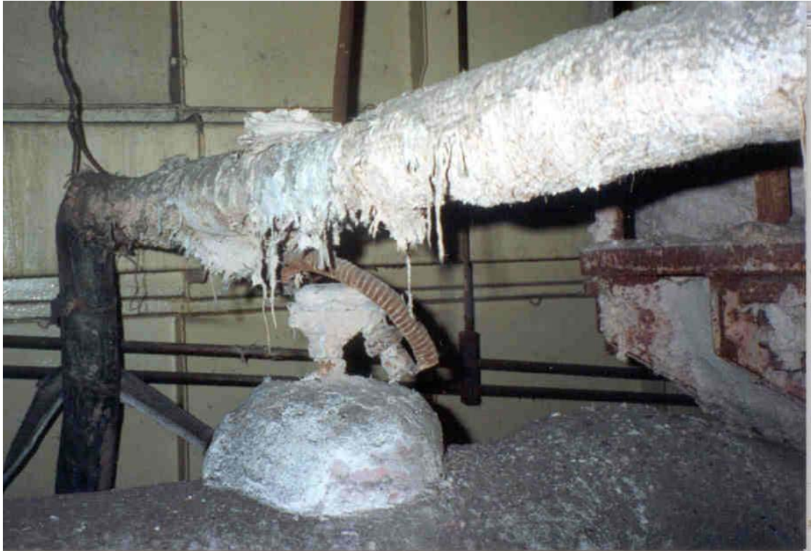
Figure 4.8 Asbestos insulation on steam pipeworks
