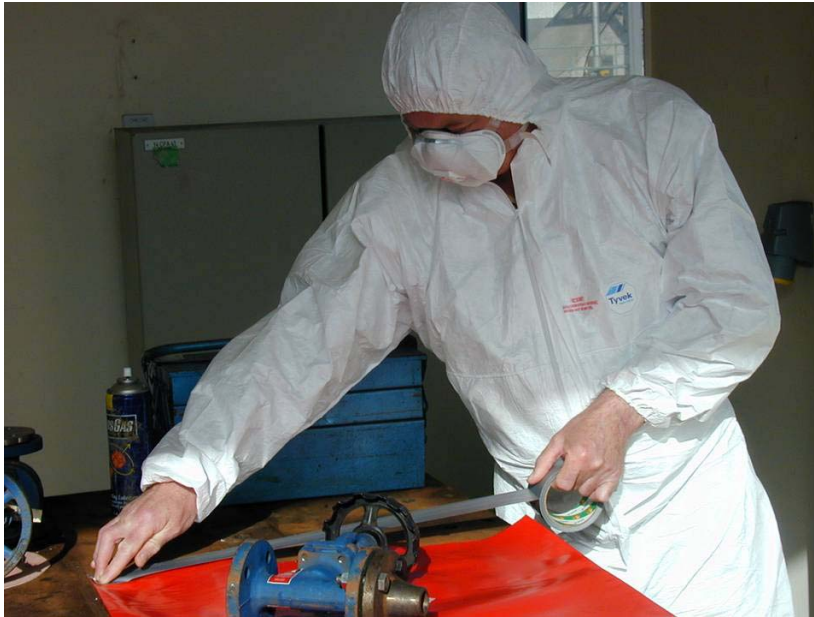
Figure 11.3 Use of tape and polythene sheeting to protect a work area before cleaning asbestos gaskets from a valve
