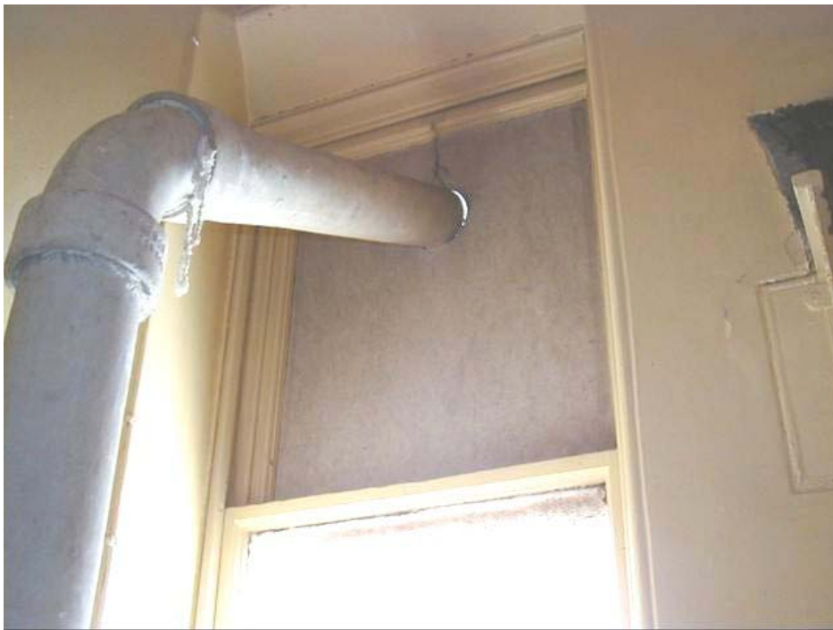
Figure 4.5 Asbestos cement flue with asbestos rope seals passing through asbestos infill panel.
