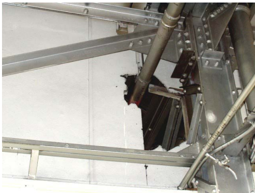
Figure 4.3 Asbestos insulating board partition wall. This example illustrates the practical difficulties in constructing a suitable enclosure and also shows the surfaces where asbestos dust may collect during the process of removal.
