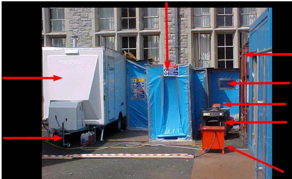
Figure 12.1 Entry to an enclosure, with arrowed from top in clockwise rotation, the baglock, the waste container, the viewing panel, the negative pressure meter, the negative pressure unit, the electrical power supply, the stock of wetting agent and the decontamination unit.
