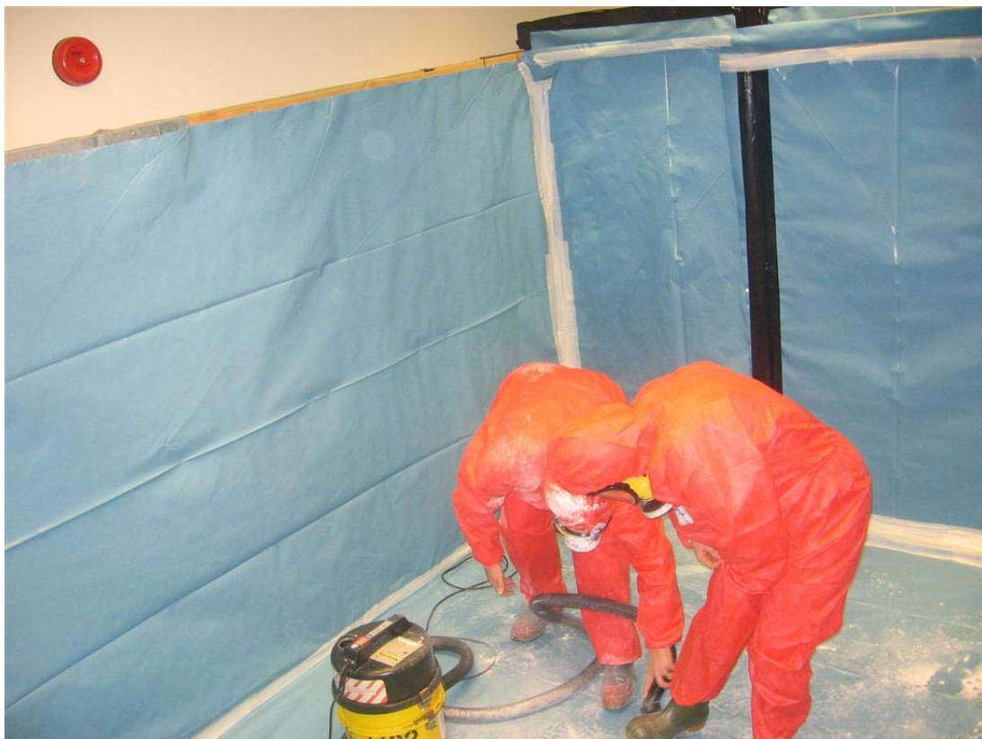
Figure 7.1 Practical training in the use of Type-H vacuum cleaners to remove simulated contamination (talcum powder). Figure provided by the UK HSE.
