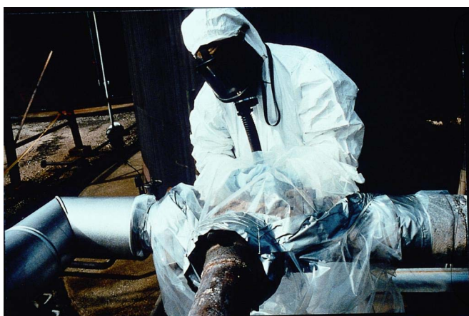
Figure 12.12 Glovebags used for controlled removal of asbestos lagging (photographs provided courtesy of INRS; copyright INRS)
